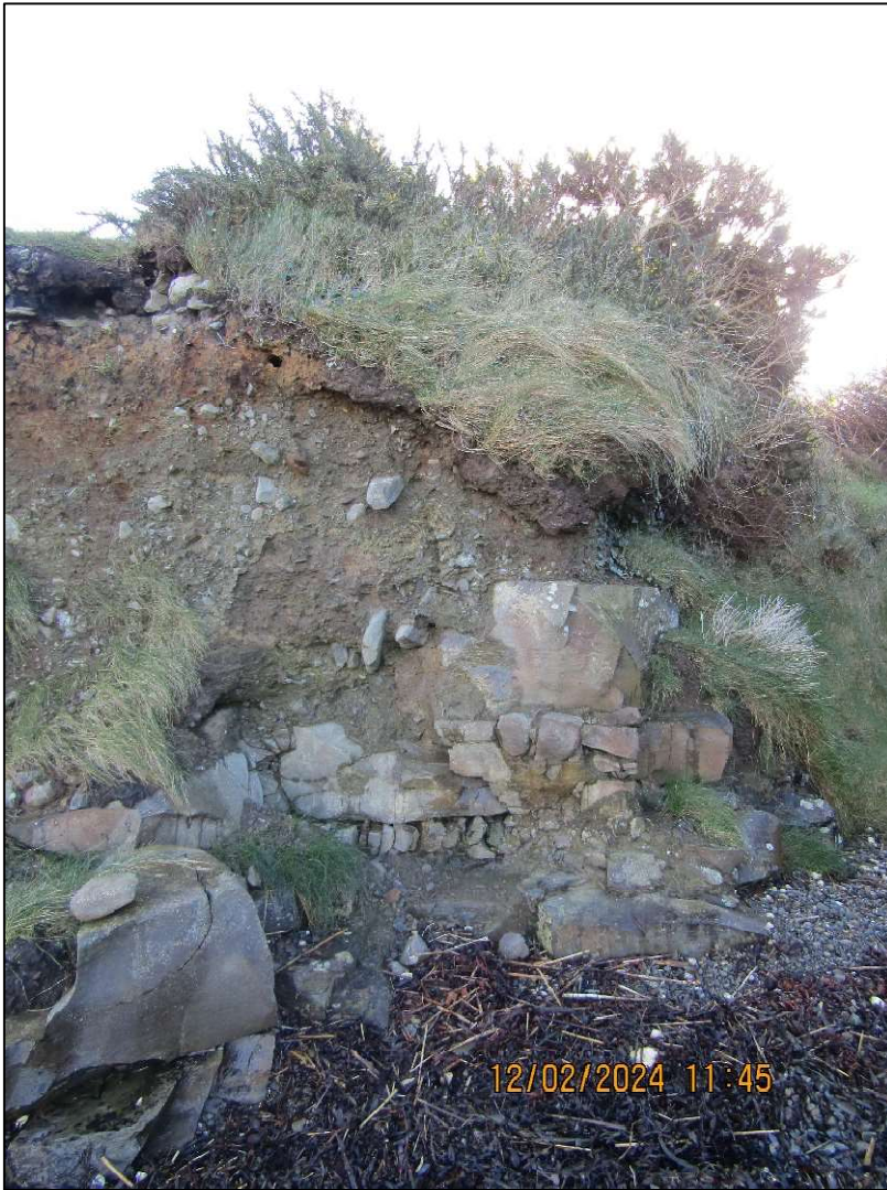
Plate 8: Earthen and stone cliffs, vegetation and side of drainage ditch, looking south.
